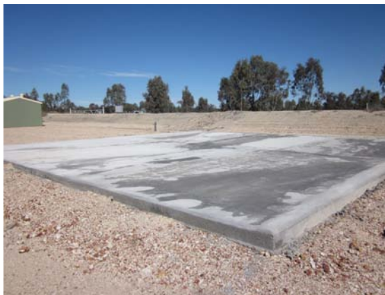
Mungindi Parthenium weed wash-down facilities with banded concrete slab and shed. Image: Jonathan Lawson
