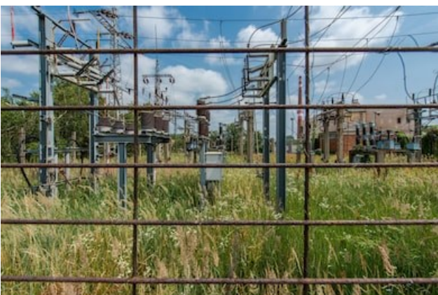
Weeds getting dangerously close to active circuits Image: Tony Cook
